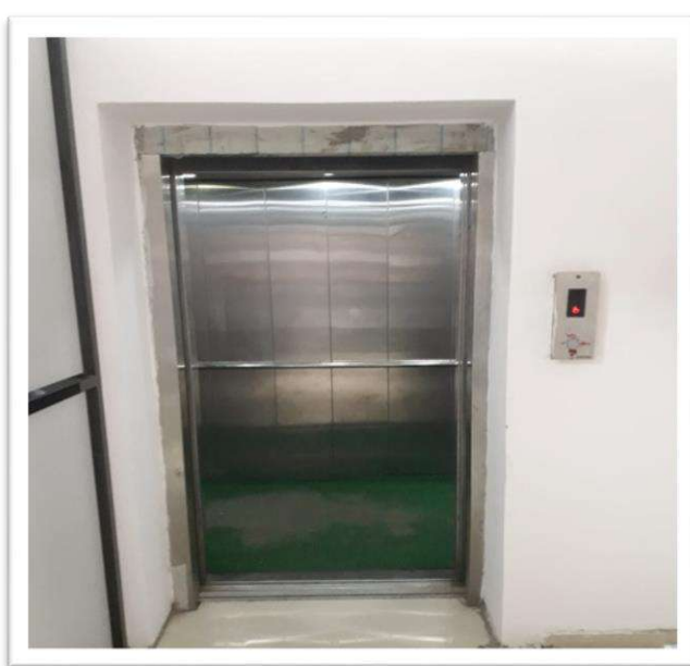
GRAB BARS IN LIFT FOR HOLD PROPERLY BY DIVYANGJAN DURING VISIT
